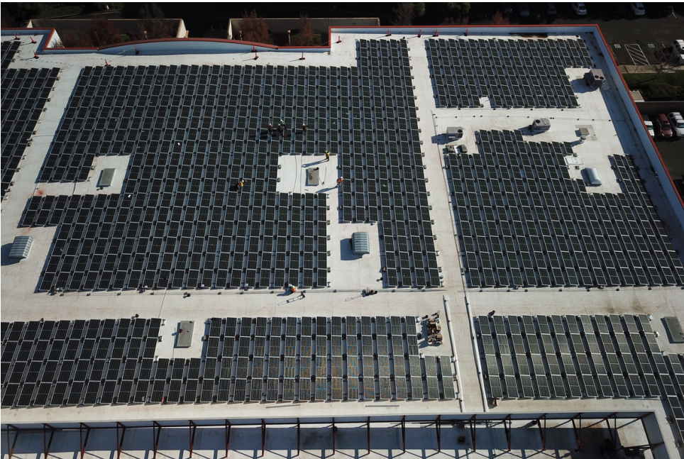
GUITTARD CHOCOLATE FAIRFIELD FACILITY, VIEW OF SOLAR PANELS
